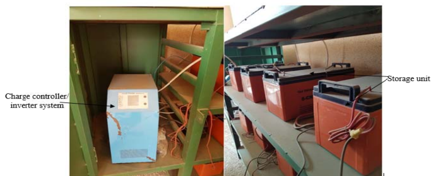
Figure 9 A storage unit and an Inverter system.
