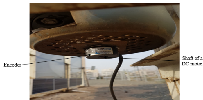
Figure 11 An encoder installed on the shaft of the DC motor
