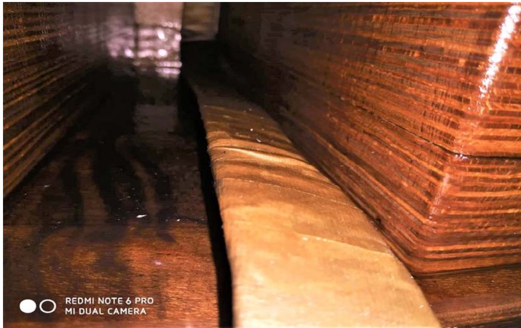
Figure 8. In internal inspection minor carbon particle find out
